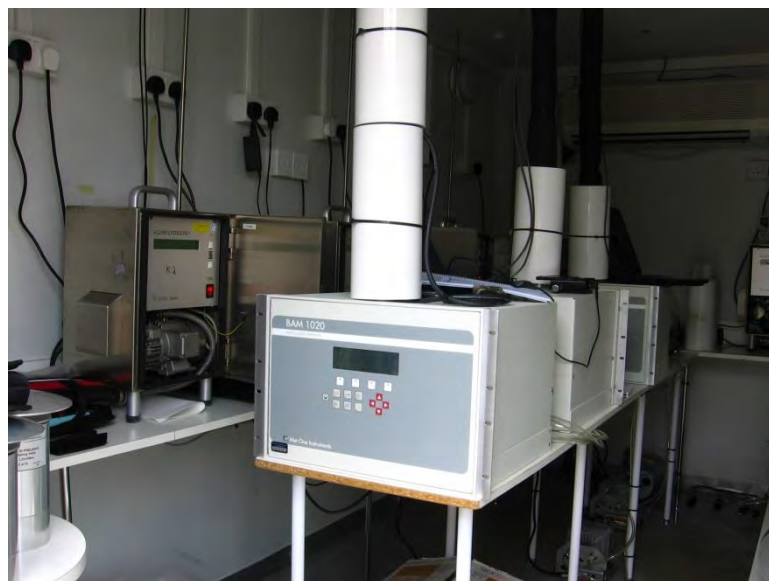
Figure 8: BAM-1020 measuring system, installed in measurement cabinet (2 performance test candidates + 1 candidate for experimental purposes (configuration of heater))
