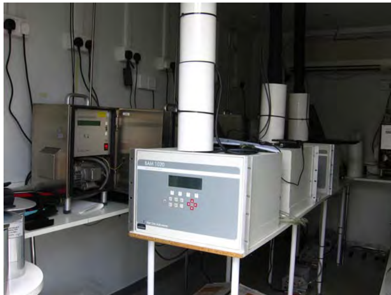
Figure 8: BAM-1020 measuring systems installed in the trailer (Two candidates included for the suitability test plus a third candidate for experimental purposes (different configuration of heater))
