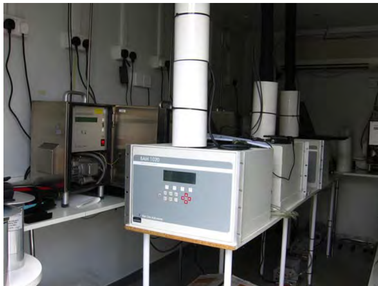
Figure 8: Measuring systems BAM-1020, installed in measurement cabinet ( 2 candidates of suitability test + 1 candidate for experimental purposes (configuration of heater)
